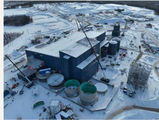
Process Plant Looking South
